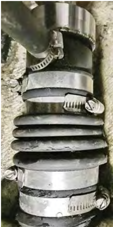
The bellows shows distinct cracks and looks worn
