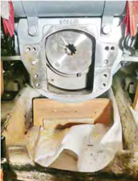
The straps led aft of the heat ex-changer and hooked to the engine mounts
