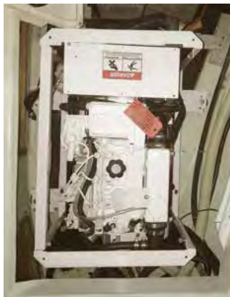
M673LD3G completely installed in compartment. Photo by Joe Rocchio
