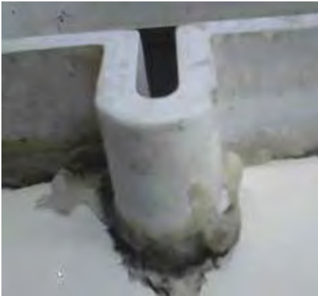
Old Sealant Under Rain Drain Lip
