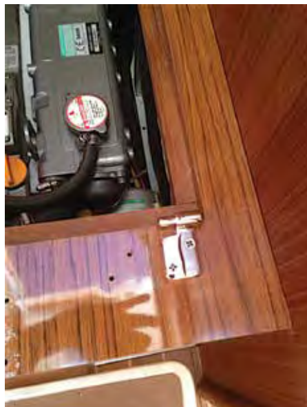
The port side pintle leaf screwed in place – showing the correct fore/aft position axially aligning the pintle structure with the gap.
