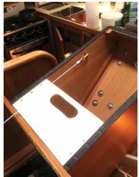
Showing the upper stair assembly tilted forward after the hinge replacement. Note the hand hole I cut in the delrin part – very helpful during the removal procedure.
